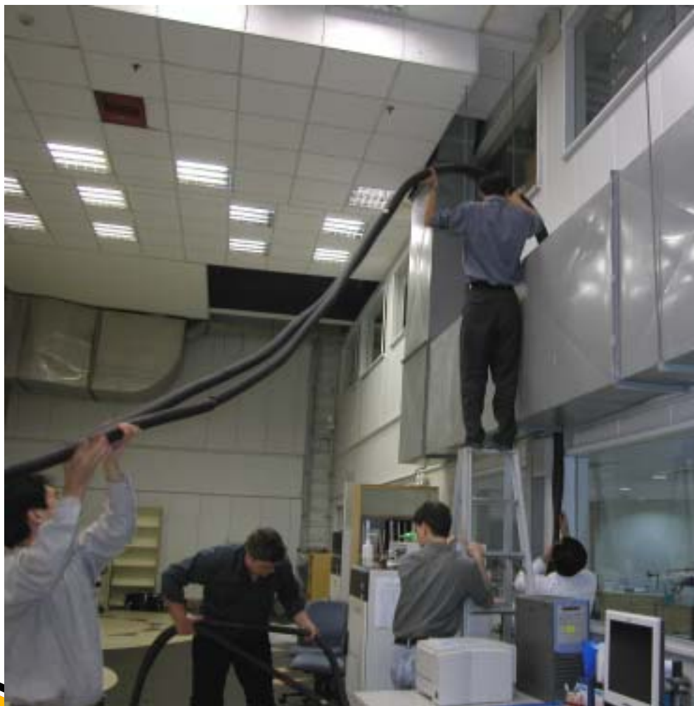
B2 NMR Room
